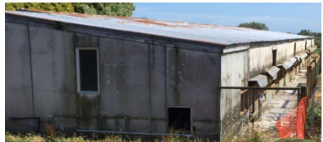
FIGURE 1: Example of a chicken shed built from asbestos containing materials
