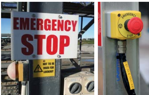
Figure 17: Emergency stop with signs
