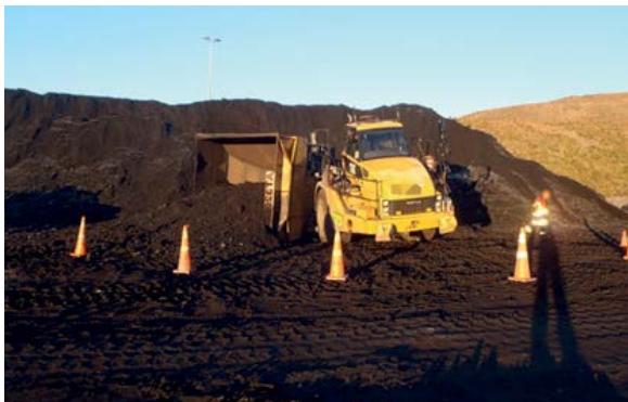
Figure 2: Vehicle overturn emergency
