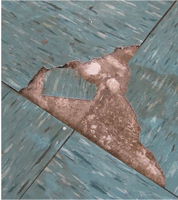
Figure 1: Floor tiles that contain asbestos can also have asbestos paper backing, or be fixed with asbestos-containing mastic
