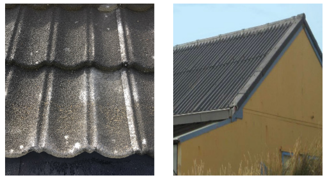
FIGURE 1: Examples of pressed metal tiles that contain asbestos and corrugated asbestos roofing material
